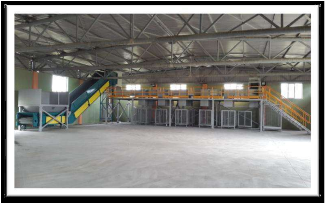
Figure 3. The applications of packaging waste collection and separation plant
