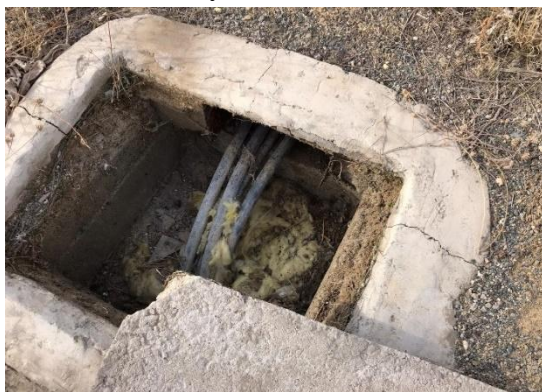
Figure 2a. Ground Heat Exchanger (GHE)
